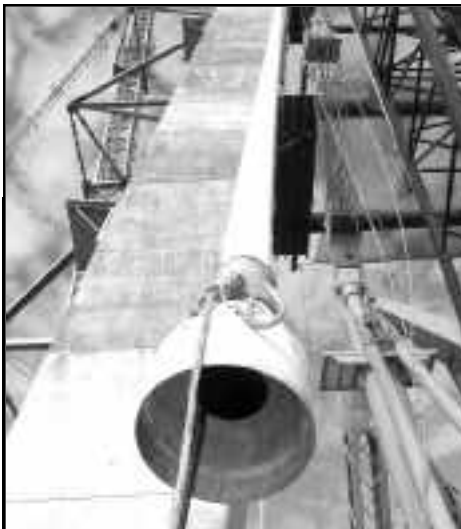
Above: Cable construction begins with the anchoring of a single master strand strung through a white, high-density polyethylene pipe. Once this master strand (as seen here behind the rope) has been anchored up on the tower and down on the bridge deck, the rest of the necessary cable strands are fed through the pipe and into the anchors.
