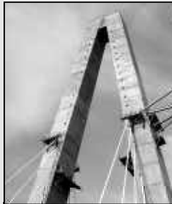
Above: Concrete was placed for the parapet wall at the top of the western tower on May 18th marking the completion of this tower. Construction for the eastern tower was completed five days later.
