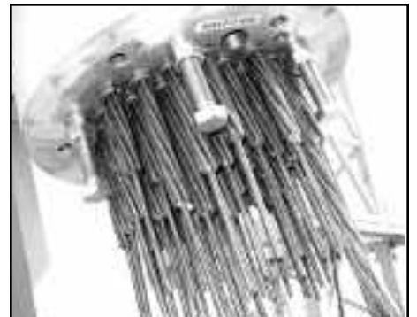
Above: The anchorage systems on the bridge deck and up in the towers hold the cable strands in the proper tension to support the bridge deck and its service load.
