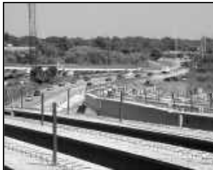
Above: With more and more girders in place, the Mount Pleasant Interchange takes shape. Pictured here are the girders for the Johnnie Dodds Boulevard (US 17) and the Coleman Boulevard ramps off of the new bridge.
